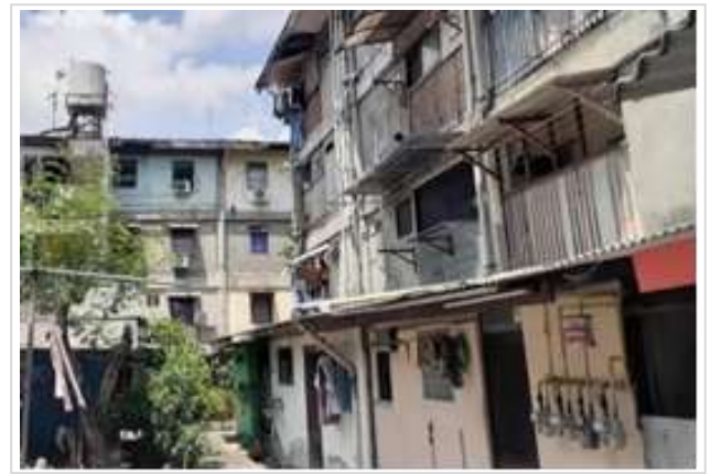
Gambar 6. Pipa air, pipa gas, outdoor AC
